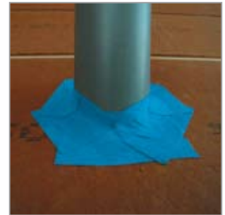
Holes for pipes Cut some roughly 10 cm long pieces from the 75 mm wide BUDAX TOP and affix to the wood fibre board or pipe in a water-tight overlapping tile formation. Alternatively, use pro clima sleeves. These should be attached with BUDAX TOP to the wood fibre board.
