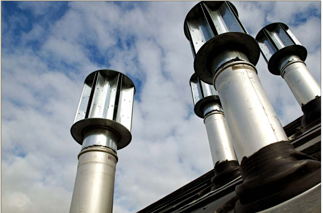
The passive stacks originate (below) in each of the wet rooms in the dwelling and rise vertically through the building and terminate above the roof (above)
