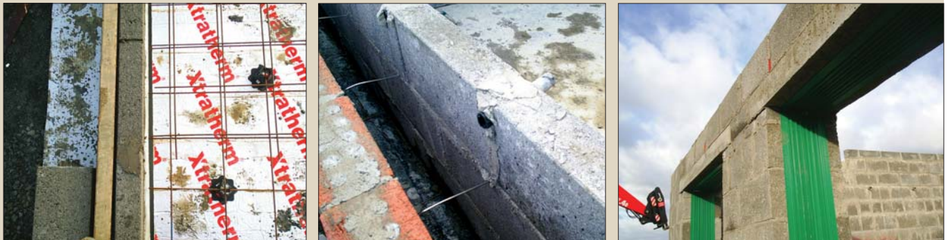
Underslab insulation in line with Perinsul block for continuous insulation (left); stainless steel cavity wall ties and inbuilt hoses for injecting full fill insulation (centre); and 200 mm cavity closers (right) are fitted to all openings in the cavity
