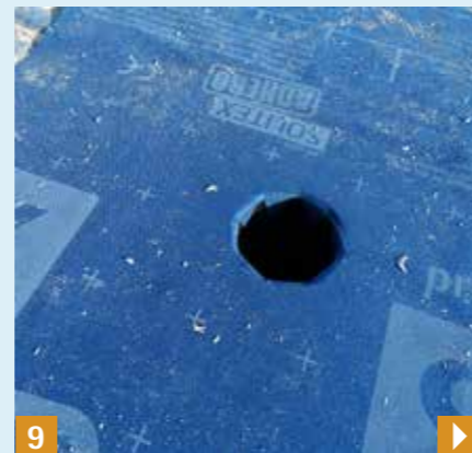
9 Practical example: remove water from the building using flexible piping installed on the underside.
