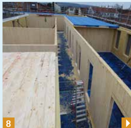
8 Avoid standing water on the membranes. If necessary, provide floor drainage or remove water by suction.
