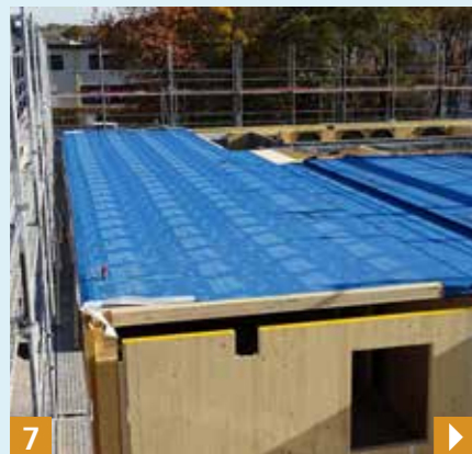
7 Stick the next membrane in place with 15 cm of an overlap onto the previous membrane.
